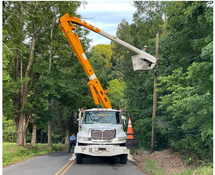
When outages occur, BTES crews work continuously until all customers' electric service has been restored.
